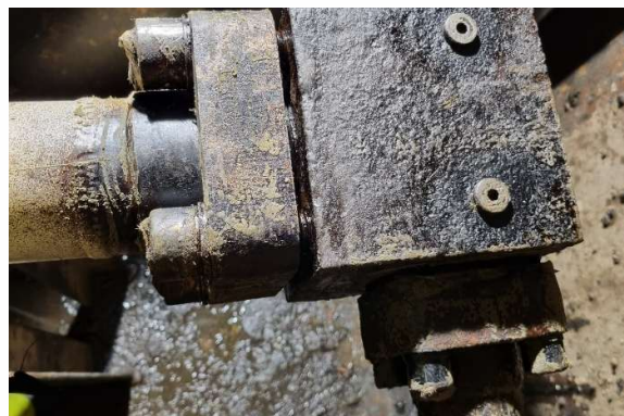
New Corroded Hydraulic Blocks & Tubing
