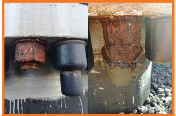
Failure of bolt caps
