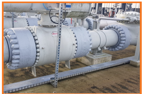
Failure of bolt caps
